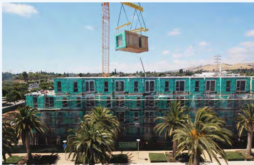
The Union Flats features 388 wood-framed modules, craned into place at a rate of 12 per day.
