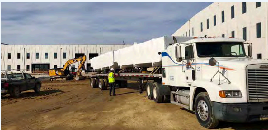
MEP racks were preassembled in a shop about 100 miles away and shipped to the site in 25ft-long 3,000-lb assemblies.
